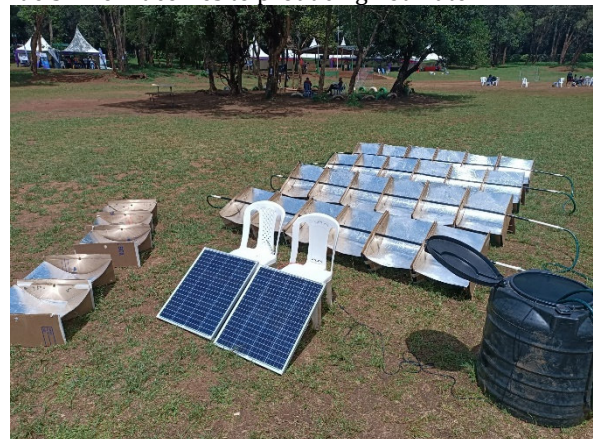
Figure 18: The collective hot water collector, growing every day with the new elements built by the scout groups
