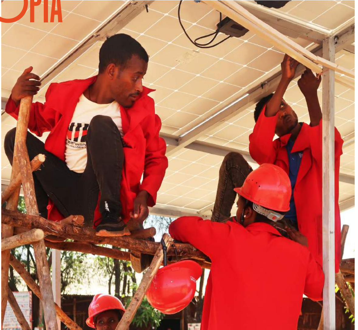
Apprentices install a PV system for a primary school in Togedro outside Bahir Dar, Ethiopia.
